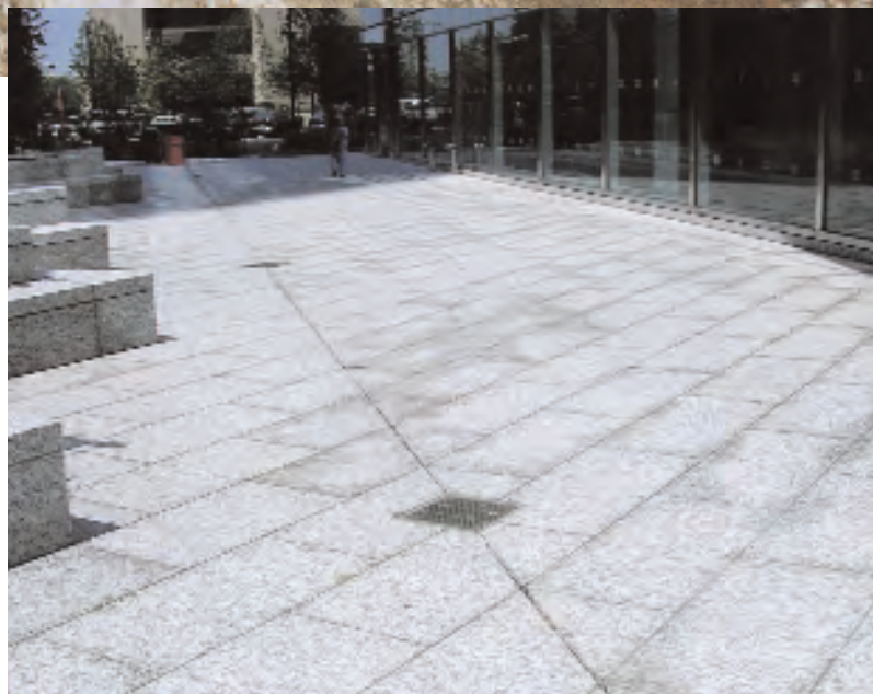
Moisture damage on exterior floor slabs.
